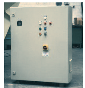
Control cabinet with frequency converter and interval cleaning
