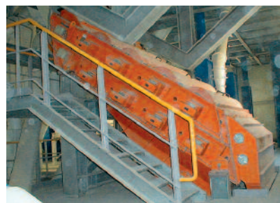
FINE SIZER in the upper part of the hopper building for limestone screening
